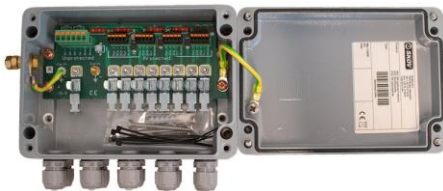
132690 DOL 199 Lightning protection
